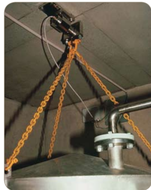
Tank suspended from KIS load cell.
